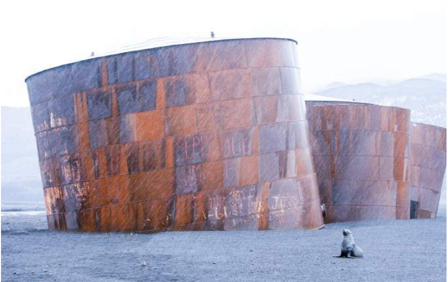
7 — Whale Oil Silos Knocked Off-Kilter by High Winds
